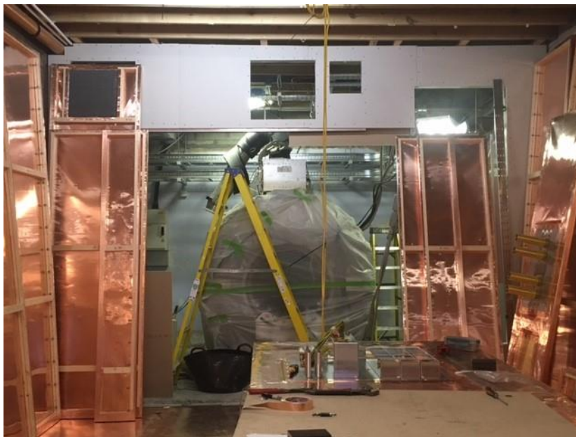
The new RF cage being installed with the magnet in the equipment room.
