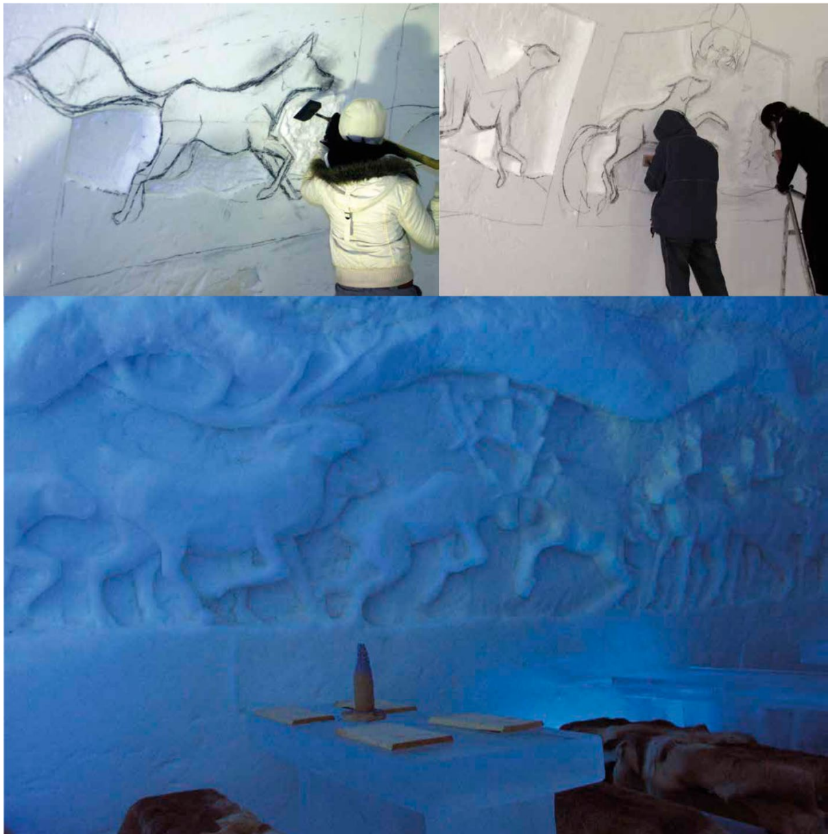
Figures 10 to 12: A group of school students work in Lainio Snow Hotel construction site together with snow and ice sculpture professionals and art education university students. At the same time, they will become familiar with an industry that counteracts emigration from Lapland, forms an alternative to
