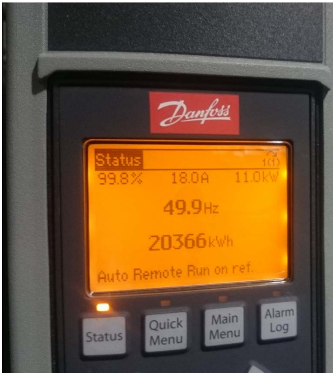
Pump Speed and Consumption before VSD Installation
