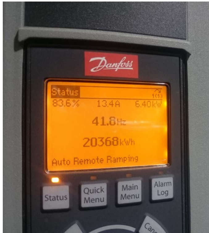
Pump Speed and Consumption after VSD Installation
