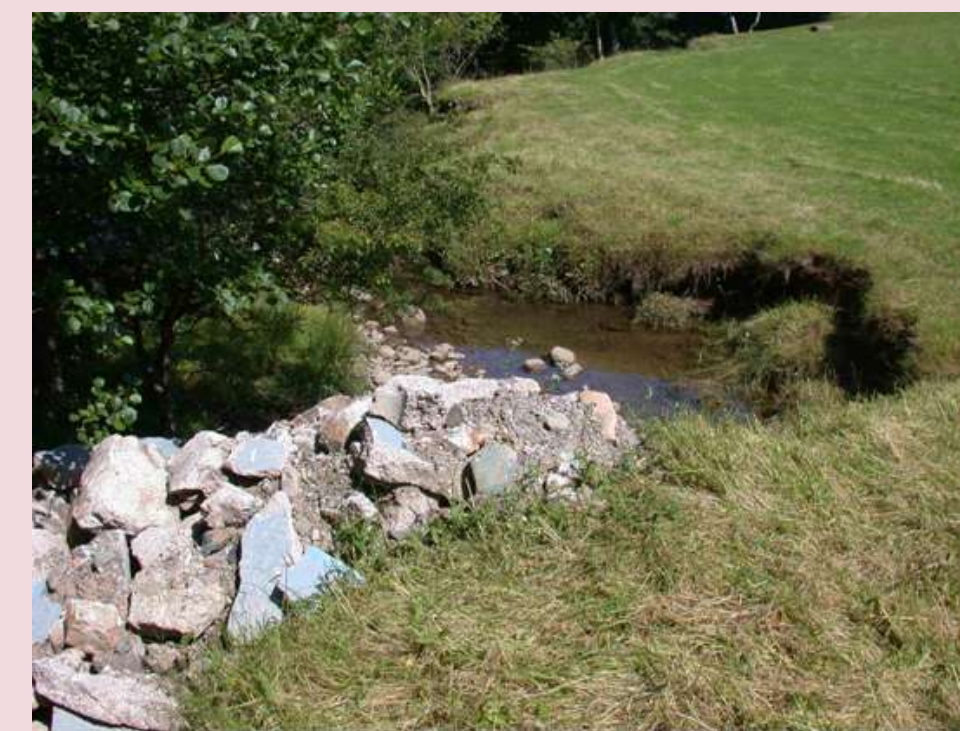
Plate 3. Ad-hoc bank protection measures on the Ehen; here a landowner has dumped waste building material in an attempt to stop bank erosion.
