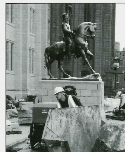
Installation of the new Robert the Bruce statue in front of Marischal College, Aberdeen. Photo by Gordon Casely
